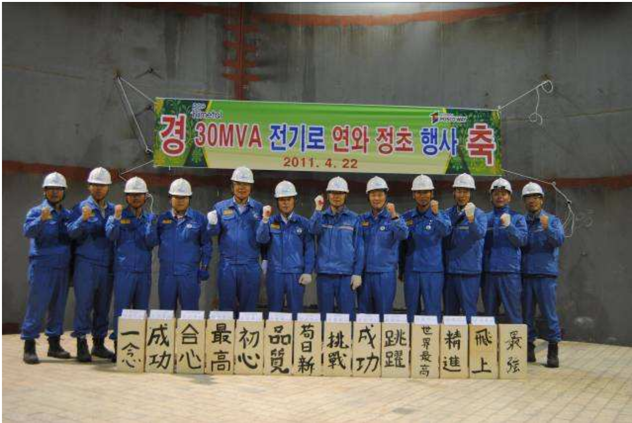
Figure 4: The banner inside the new POS HiMetal SiMn furnace reads: “Congratulation Ceremony for successful lining installation of 30MVA SAF”
