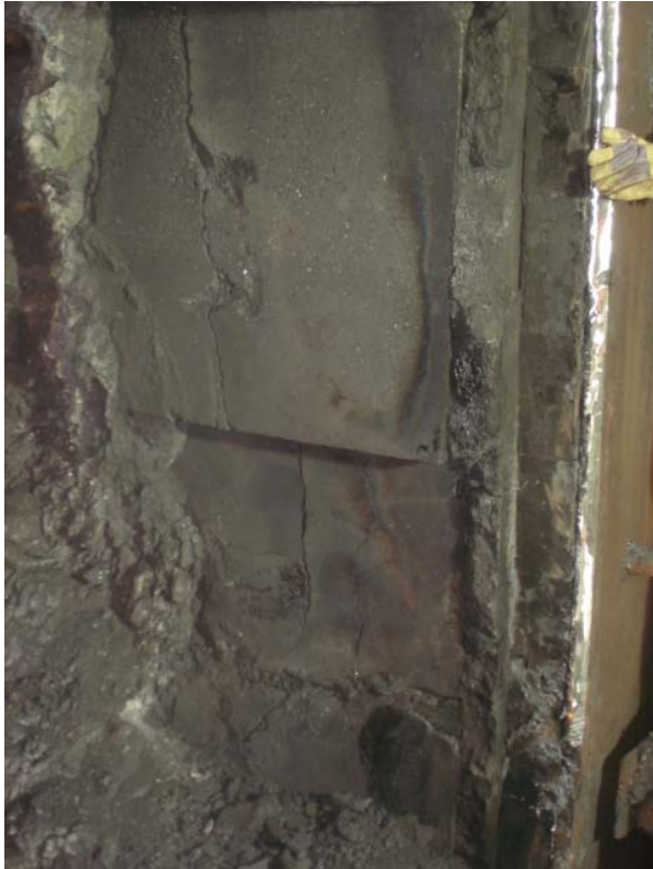
Figure 2. Typical wear and cracks in a micropore carbon large block hearth wall, also referred to as “Ring Crack” (In this case after an 8 year campaign).
